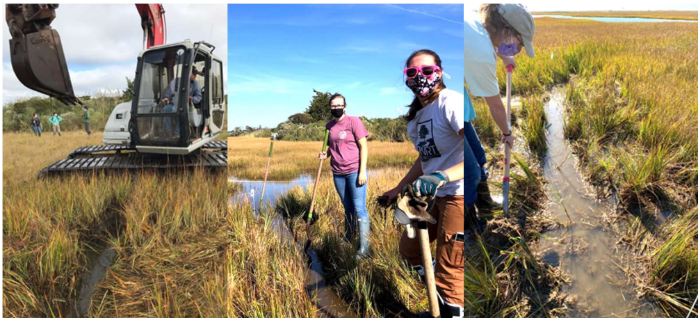
Figure 7. Creation of runnels at Ocean View Farm. Top and Bottom Left: Bristol County Mosquito Control operator creates a runnel with a low-ground pressure excavator. Bottom Center: Staff and volunteers hand-dig a runnel. Bottom Right: Wenley Ferguson hand digs a runnel. Photos: R. Jakuba, A. Besterman, W. Ferguson.
